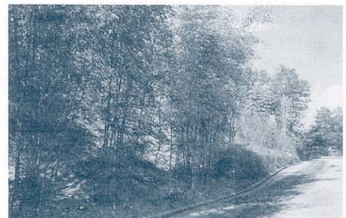
A stand of large bamboos can catch debris and support the base of a slope
