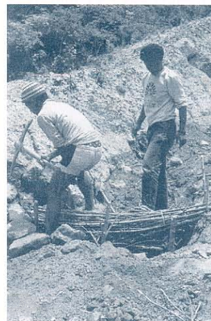
Backfill around the check dam and compact the soil with foot pressure
