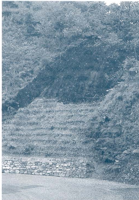
A revetment toe wall is protected by grasses planted on the slope above
