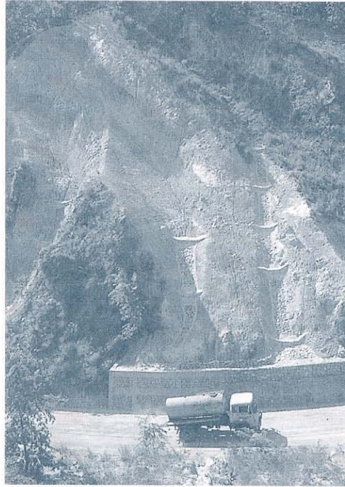
Small check dams at frequent intervals are effective, even in very steep gullies
