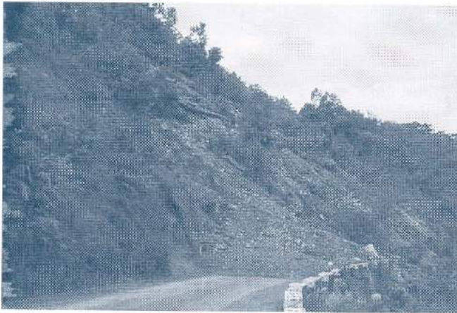
Shallow planar failures on long steep slopes can give rise to large volumes of debris. Although the debris in this example is about 5m deep, the depth of the failure itself is less than 1m
