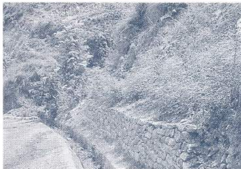
Shrubs planted above a toe wall catch loose debris moving down the slope
